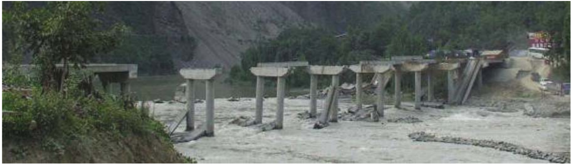
Fig. 4 Damage scenario of the 10-span bridge under construction during the earthquake
