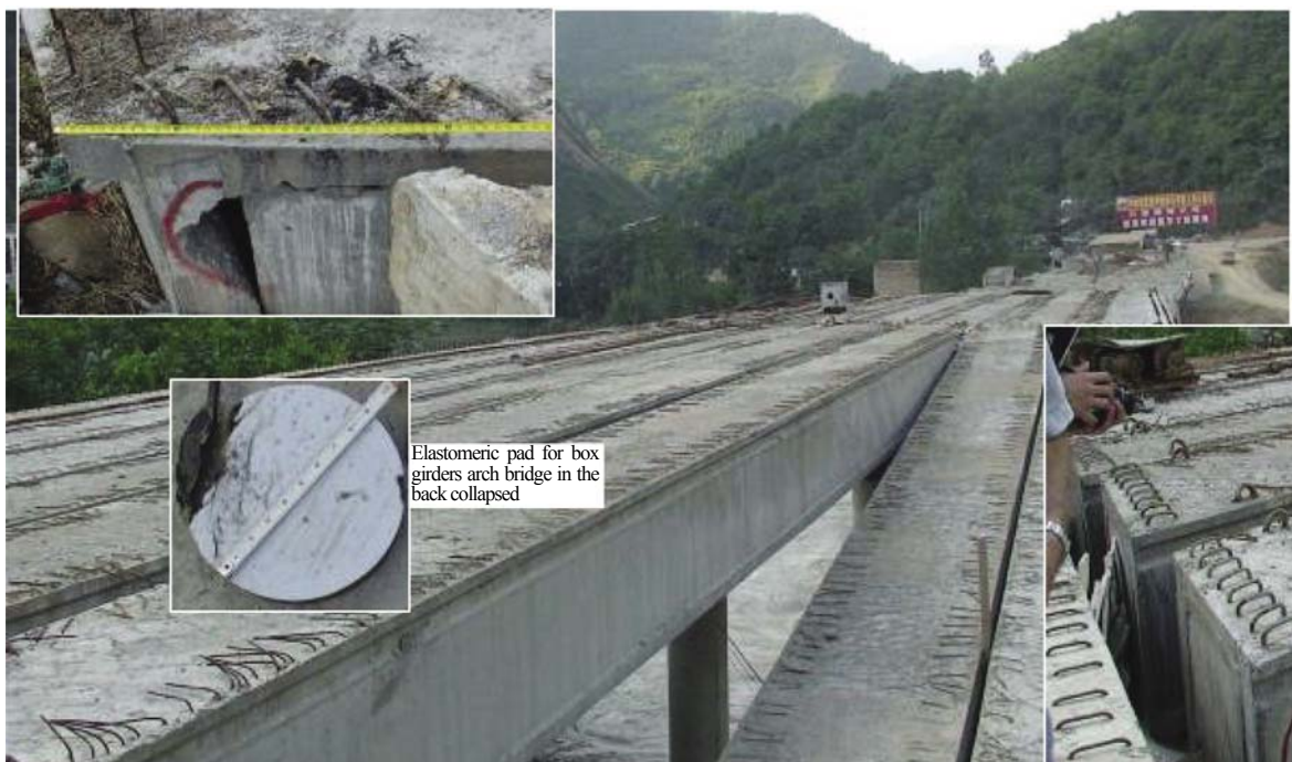
Fig. 5 Damage to the 10-span bridge under construction
