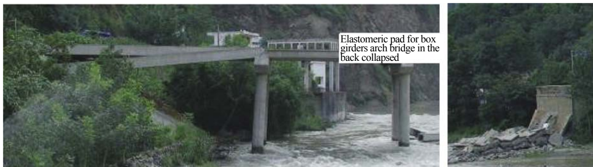
Fig. 3 Collapse of the old three-arch bridge
