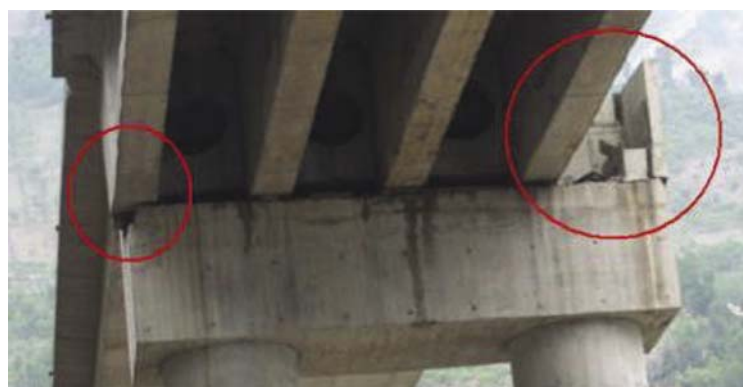
Fig. 19 Damage at Bent 9
