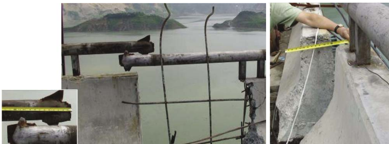
Fig. 11 Longitudinal and transverse offset of bridge deck
