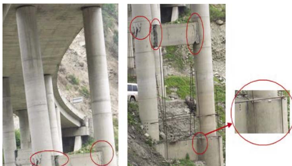
Fig. 18 Damage at Bent 3
