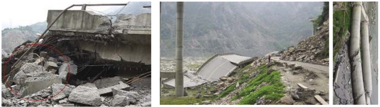
(a) Column shear and flexural failure
