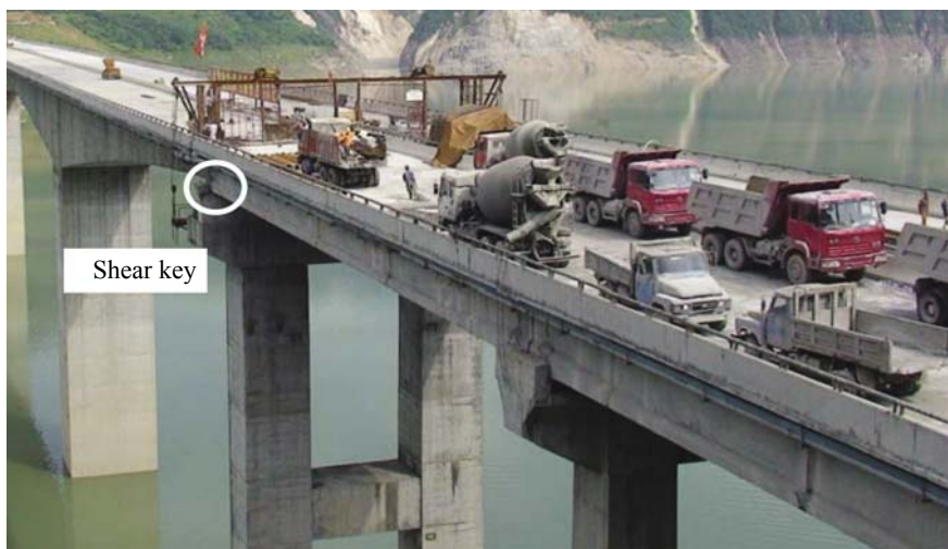
Fig. 12 Shear key failure
