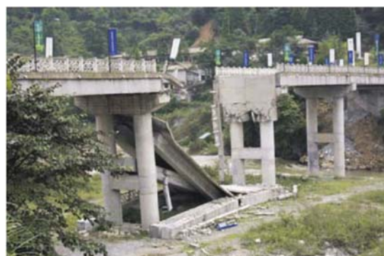
Fig. 7 Unseating of superstructure (Yuan et al. , 2008)
