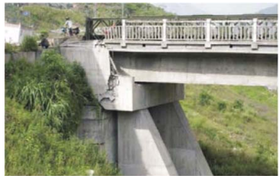
Fig. 10 Abutment damage (Yuan et al. , 2008)
