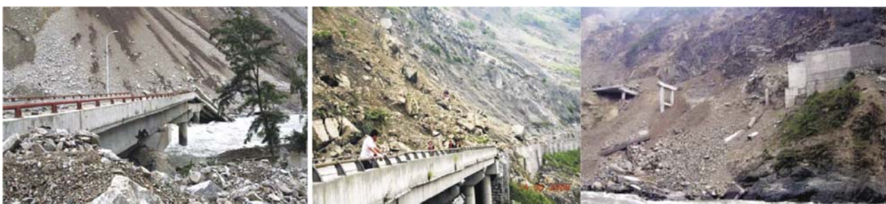
Fig. 3 Three damaged bridges in Duwen Roadway induced by landslide or rockfall (Yuan et al. , 2008)
