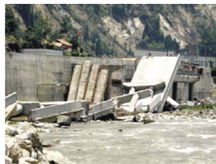
Fig. 2 Collapsed Gaoshu Bridge (Yuan et al. , 2008)
