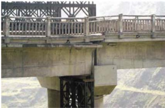
Fig. 9 Dislocated of superstructure (Yuan et al. , 2008)
