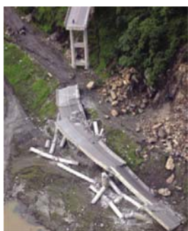
Fig. 14 Collapse of five curve span
