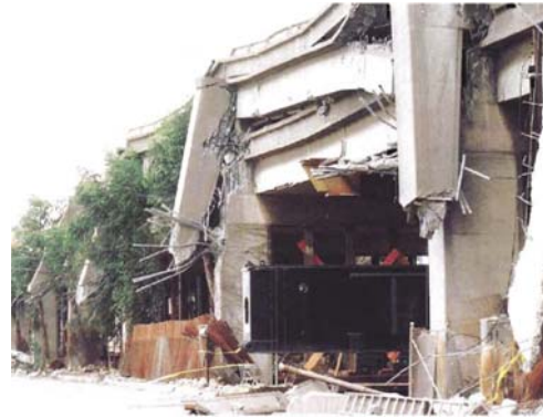
Fig. 19 Cypress viaduct (Housner et al. , 1990)
