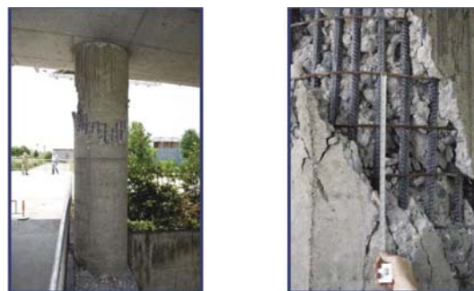
Fig. 15 Shear failure of column of Mianyang Airport viaduct (Chen et al. , 2008)
