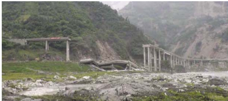
Fig. 11 Collapsed Baihua Bridge (Li et al. , 2008)
