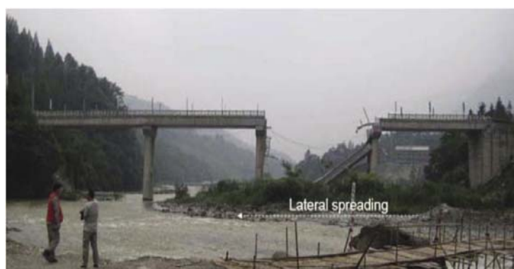
Fig. 6 Gaoyuan Bridge nearby fault trace (Chen, 2008)
