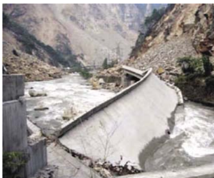
Fig. 12 Collapsed Yuzixi Bridge (Yuan et al. , 2008)
