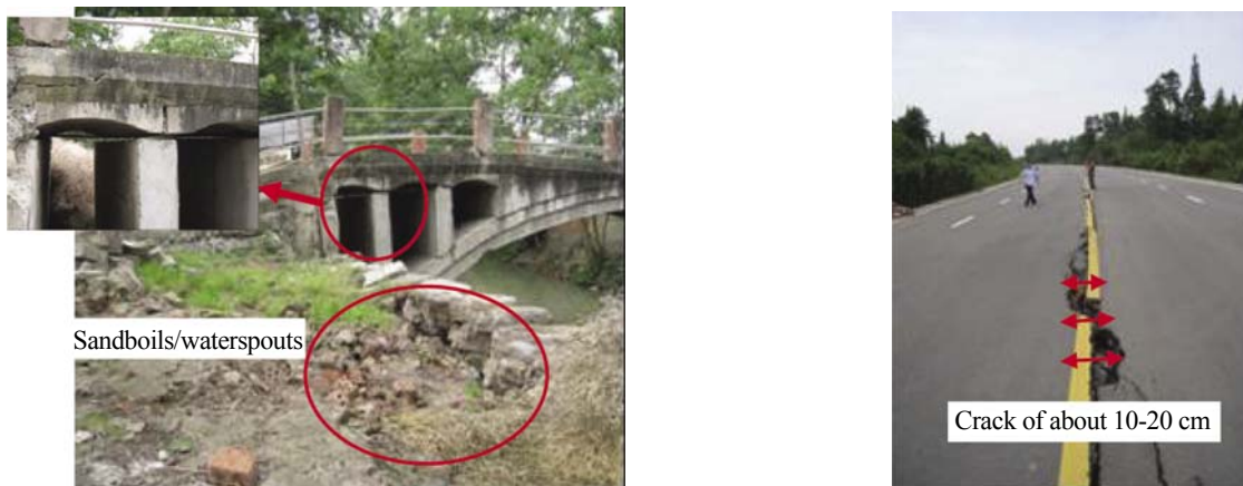
Fig. 17 Liquefaction-induced destruction to bridge (left) and road (right) (Photo by ZZ Cao and FC Meng)
