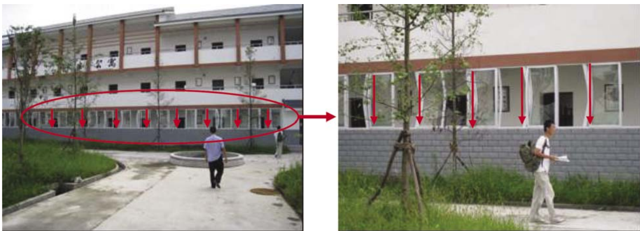
Fig 16 Liquefaction-induced settlement/differential settlement caused the deformation of the window frames in Zhongxing Middle School in Dujiangyan City (Photo by LW Chen)
