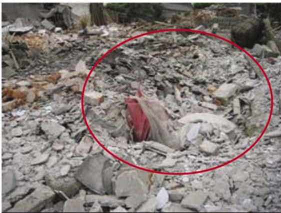
Fig. 9 Large pit of about 3 m in diameter destroyed a house (Photo by ZZ Cao)
