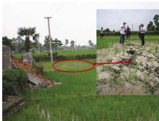
Fig. 3 Liquefied site with a high water ejection of about double the height of the wire pole and a visible ground failure (Photo by WM Wang)
