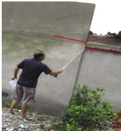
(a) Differential settlement caused by liquefaction
