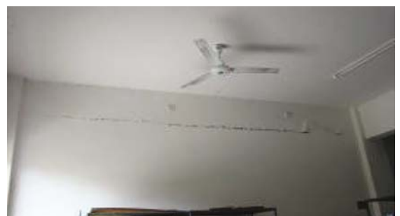
(d) Cracks in infill wall below the beam on the ground floor
