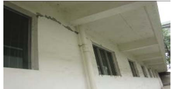
(a) Infill wall # I cracked at the upper level of windows
