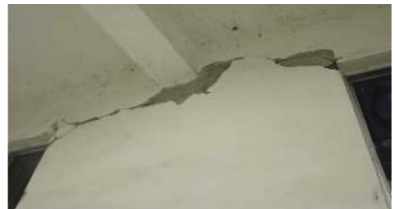
(b) Infill wall # II cracked at the upper level of windows, view is from inside the building
