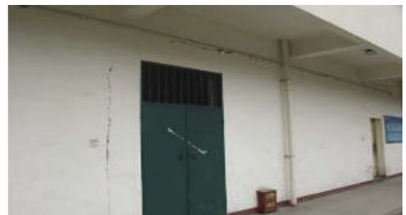
(c) Cracks between infill walls and columns on the ground floor
