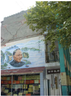
Fig. 14 Severely damaged three-story masonry school building (0.05g/0.20g)
