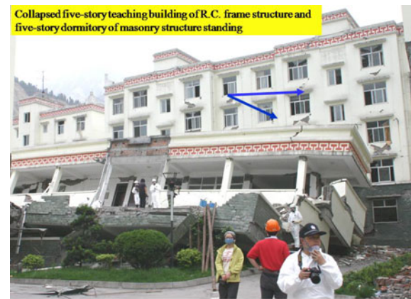
Fig. 21 Totally collapsed laboratory building (0.1g/1.0g)
