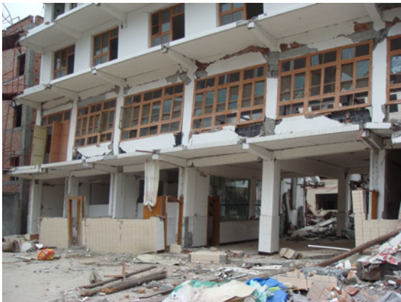
Fig. 23 Severely damaged four-story RC single-bay frame single span hospital building (0.1g/0.4g)
