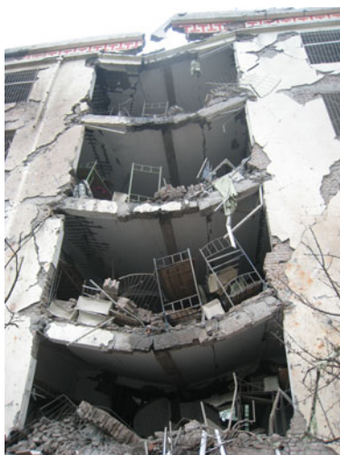
Fig. 11 Large deflection of floor formed with cast-in-situ RC beams and slabs (0.1g/1.0g)
