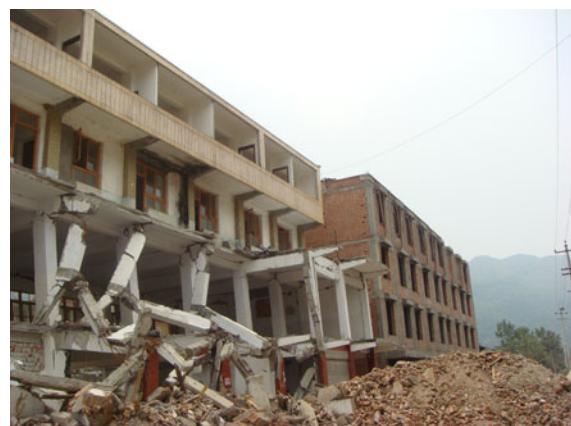
Fig. 22 Damage to two nearby buildings (0.1g/0.4g)
