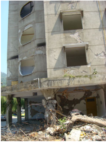
Fig. 6 Damaged RC bottom frame structure (0.1g/0.4g). Note: (0.1g/0.4g) = (specified PGA/estimated PGA)
