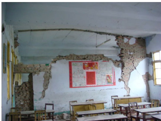
Fig. 15 Collapse of transverse wall (0.05g/0.20g)
