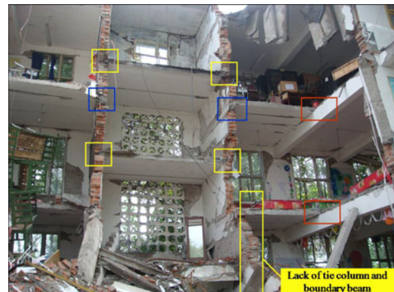
Fig. 27 Collapsed stair shaft of a three-story school building in Mianzhu County (0.1g/0.3g)
