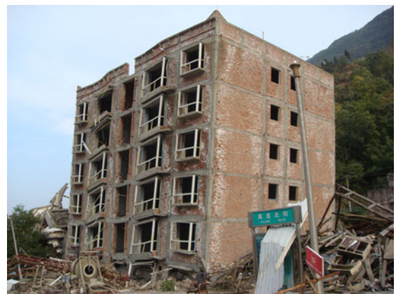
Fig. 17 Two bottom stories collapsed and five upper stories remained standing, Beichuan County (0.1g/1.0g)
