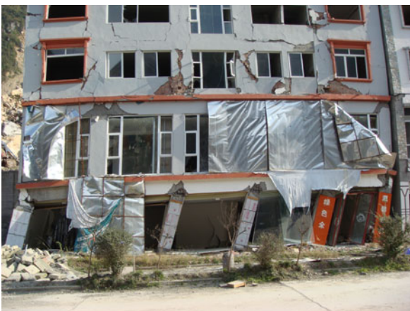
Fig. 8 Damaged masonry building with two-story RC bottom frame structure (0.1g/1.0g)
