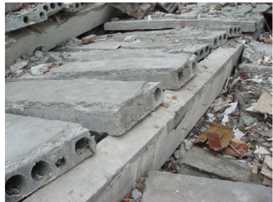
Fig. 12 Collapsed pre-cast RC floor slabs (0.1g/0.2g)
