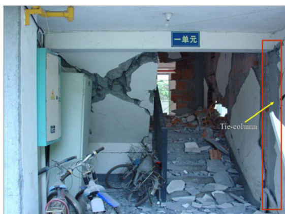
Fig. 28 Six-story masonry residence building remained stable with a severely damaged stair shaft (0.1g/0.3g)
