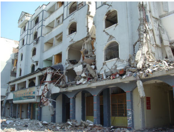
Fig. 7 Damaged upper walls of masonry building with RC bottom frame structure (0.1g/0.4g)
