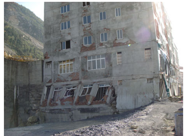
Fig. 5 Bottom frame structure severely damaged due to failure of slope wall
