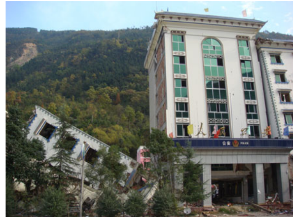
Fig. 25 Collision between an office building and apartment buildings in Beichuan County (0.1g/1.0g)
