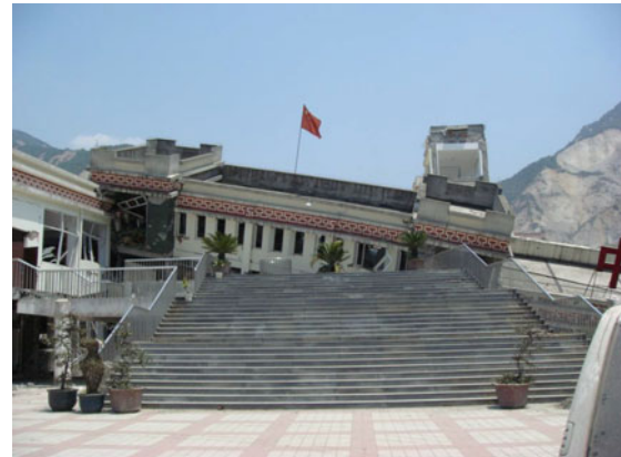
Fig. 20 Partially collapsed teaching building (0.1g/1.0g)
