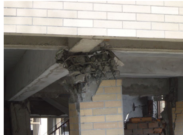
Fig. 9 Plastic hinges on top of a column (0.1g/0.3g) (Photo from Yao Qiulia)
