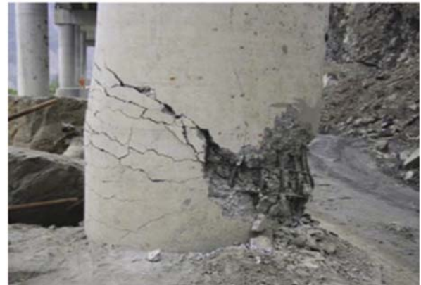
(b) Shear failure
