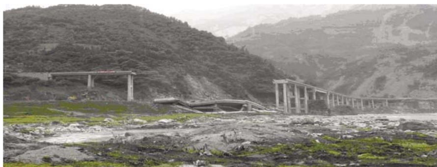
Fig. 5 Failure of the Baihua Bridge
