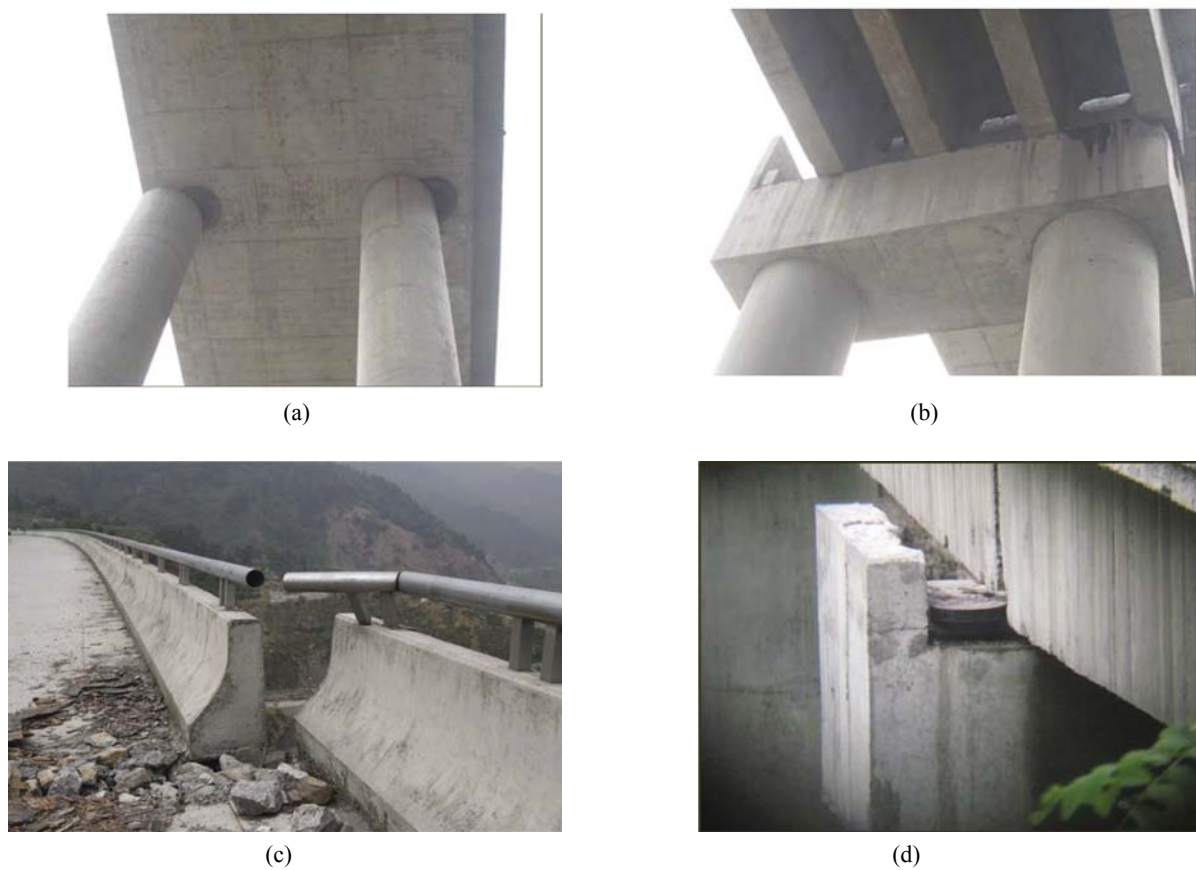
Fig. 13 Sliding between the top of the laminated-rubber bearing and the bottom of the girder
