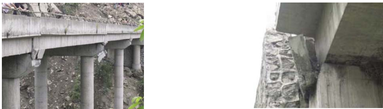
Fig. 14 Typical shear key damage
