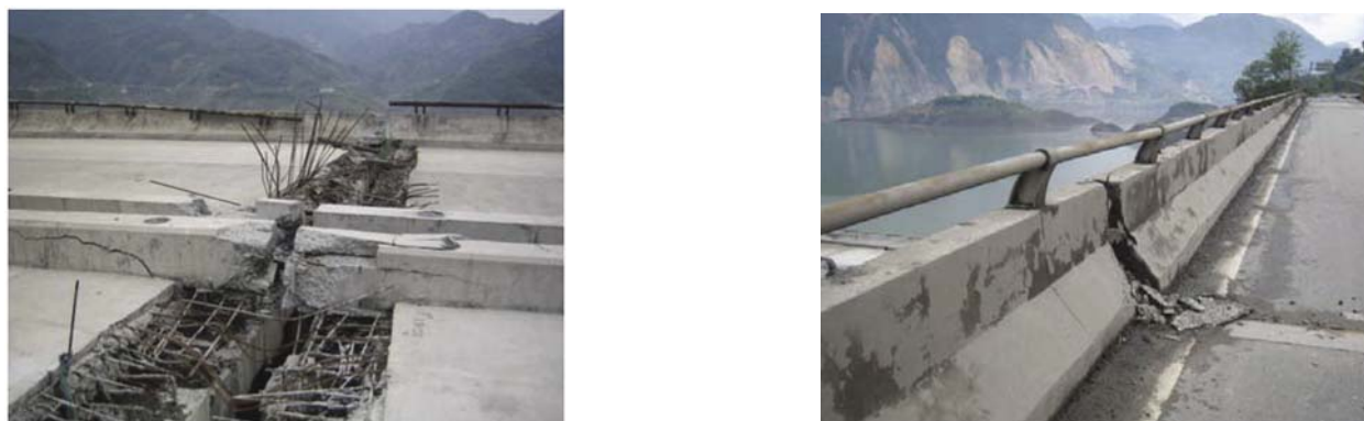
Fig. 15 Typical expansion joint damage
