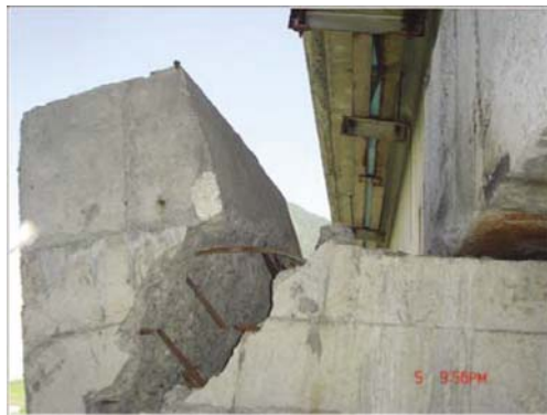
(a) Shear key damage
