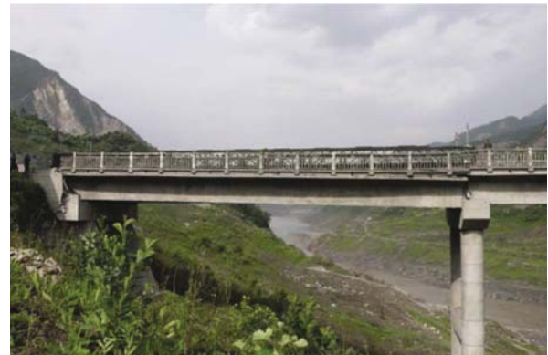
(b) Collapse of the bearing of girder at pier 1
