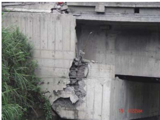
(a) Lateral displacement of girder at abutment
