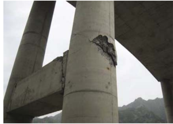
Fig. 6 Column joint failure
