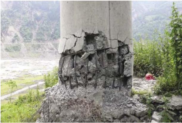
(a) Confinement failure
