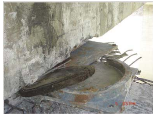
(b) Bearing damage
