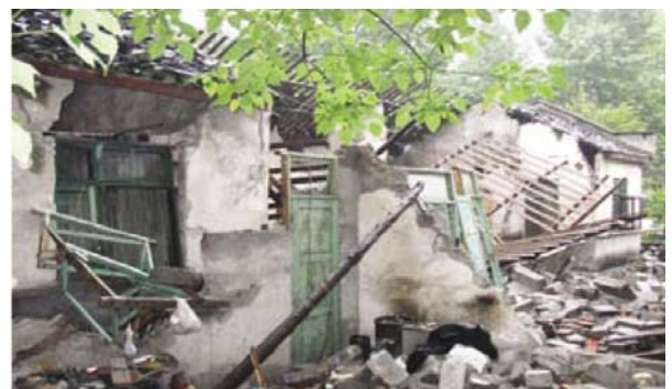
Fig. 4 Brick-wood residential building in Yangcha Village (Group A, collapsed)
