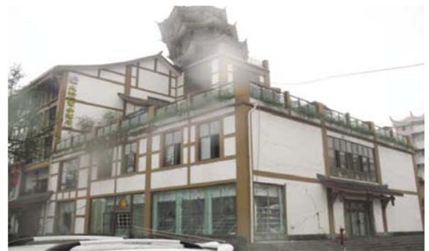
Fig. 17 Tiandiren Hotel (Group C, top building collapsed)
