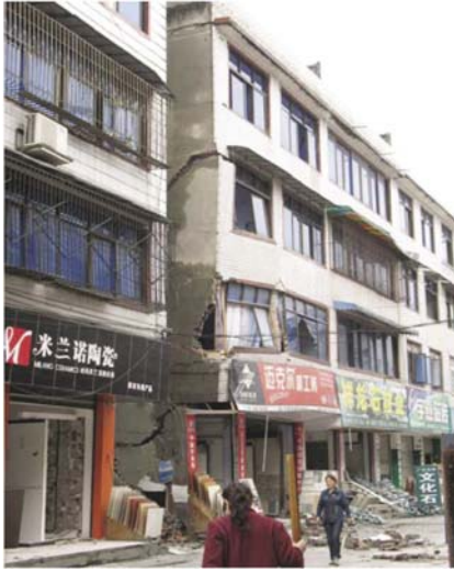
Fig. 12 Masonry building with a ground story of RC frame in Kuiyuanxijie District (Group B, seriously damaged)
