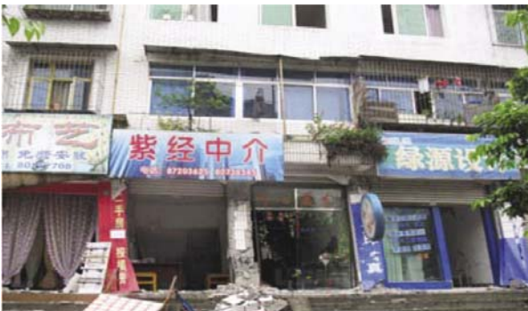
Fig. 8 Masonry building with a ground story of RC frame structure in Hehuachi District (Group B, seriously damaged)
