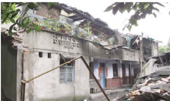
Fig 2 Two-story brick-wood residential building in Hongzhuangjie District (Group A, roof collapsed)
