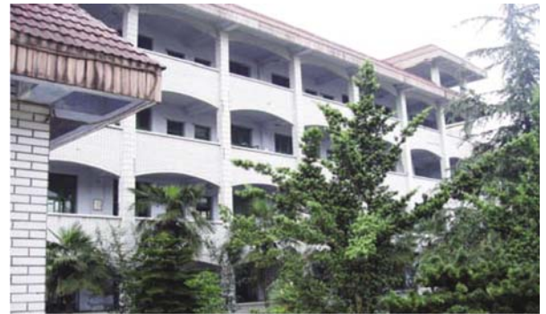
Fig. 16 Masonry building of Tazhonglianzhong School (Group C, moderately damaged)
