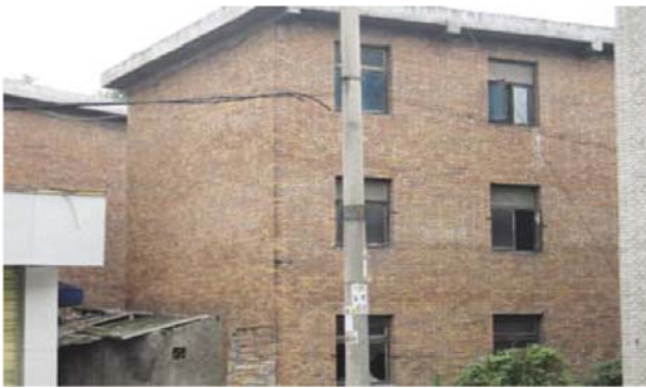
Fig. 6 Masonry building in Kuiguang Street (Group B, moderately damaged)
