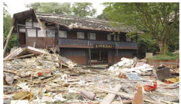
Fig. 5 Timber structure in Erwangmiao scenic spot (Group A, roof damaged, inclined)
