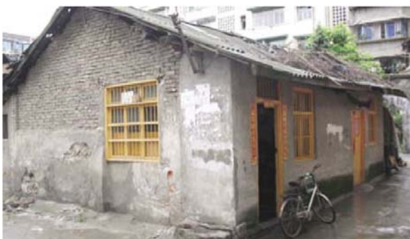
Fig. 3 One-story brick-wood hut (GroupA, moderately damaged)
