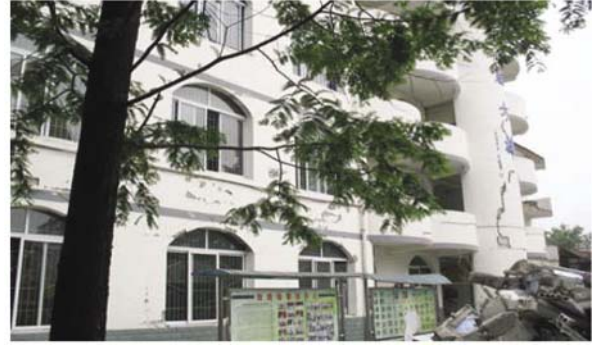
Fig. 15 Masonry laboratory of Juyuanzhen Middle School (Group C, seriously damaged)
