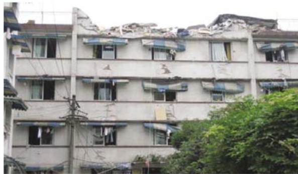
Fig. 7 Masonry structure, students' dormitory of Chengdu University (Group B, top collapsed)
