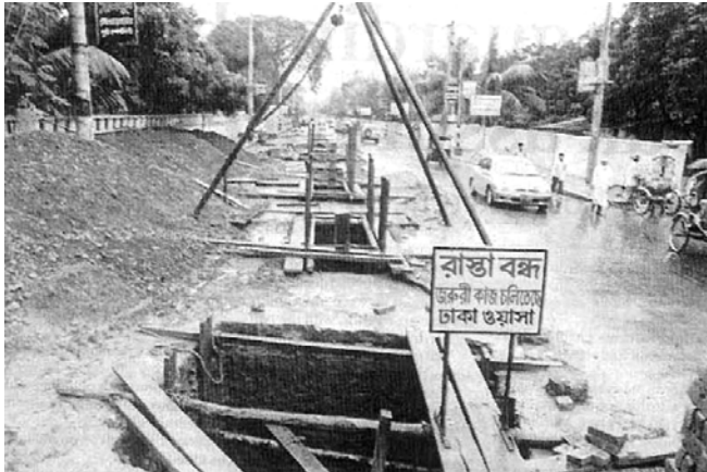
Picture-5.9 Development Work during Rainy Season Leads to Water Logging
