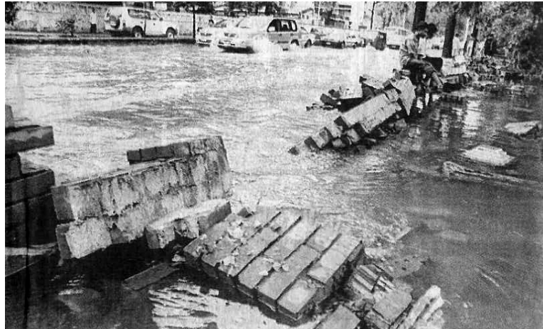
Picture-6.4 Water Logging due to Heavy Rainfall in Dhaka city Damage Structure
